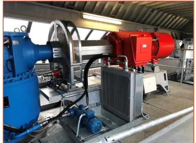
Leitner rope way overhead drive
