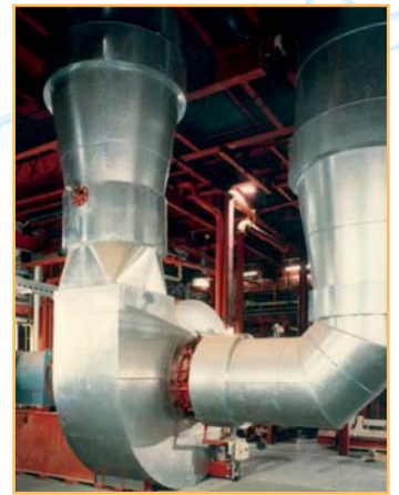
Compressor and ventilator shaft seal
