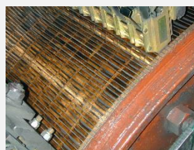
P43 – Spark burn at bar edges
