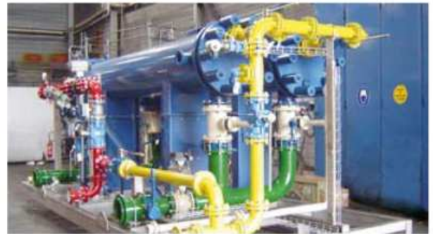
Dilution Skid – 96T/h 84% H 2 SO 4
